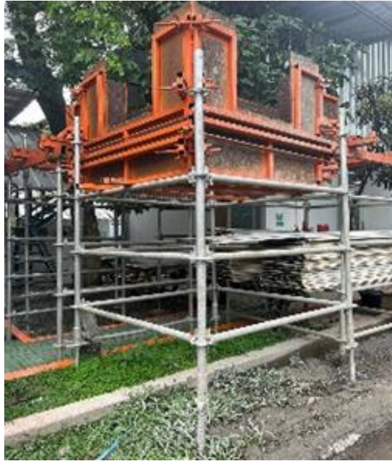
Gambar 4. Perancah Ringlock Scaffolding System
