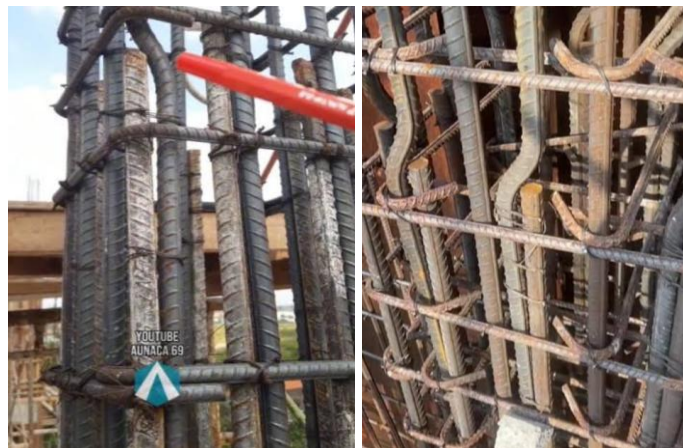
Gambar 5. Joint Rebar Tanpa Coupler
